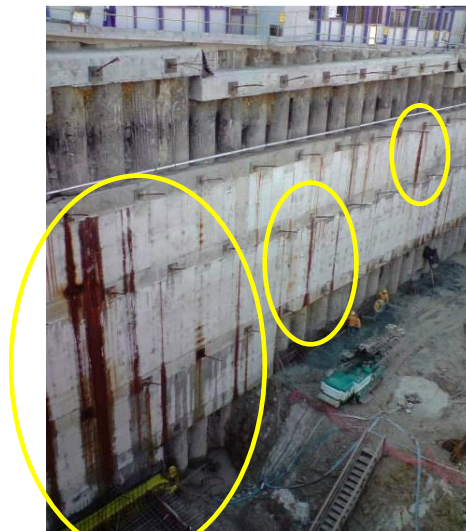
Figure 20. Seepage through ground anchor's heads.
