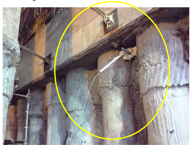
Figure 19. Major water loss due to an unpredicted flow path.
