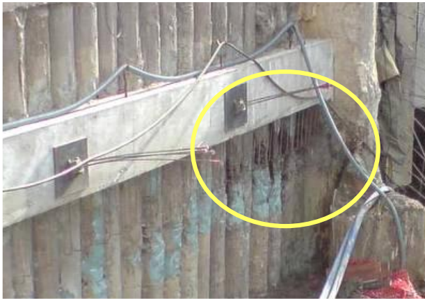
Figure 21. Example of concrete fault in the bored secant piles.
