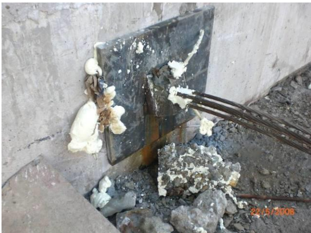
Figure 17. Ground anchor head treated with polyurethane expansive foam.
